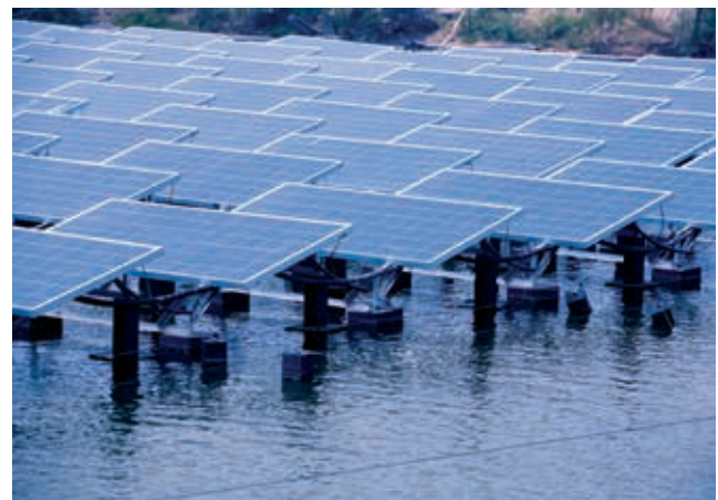
General View of the Eshkol installation
