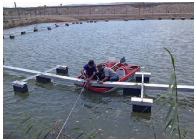
Installation Process: The installation of the floating tension ring that hold the stainless steel wire grid
