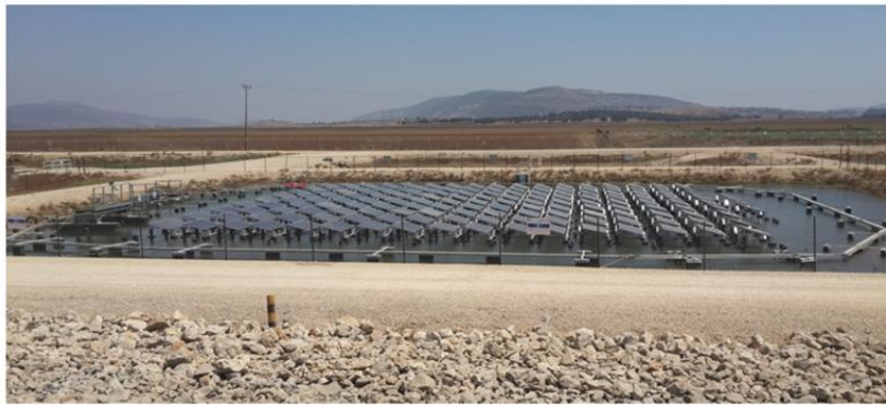
The Solaris Synergy Solar on Water installation in Eshkol reservoir, Israel
